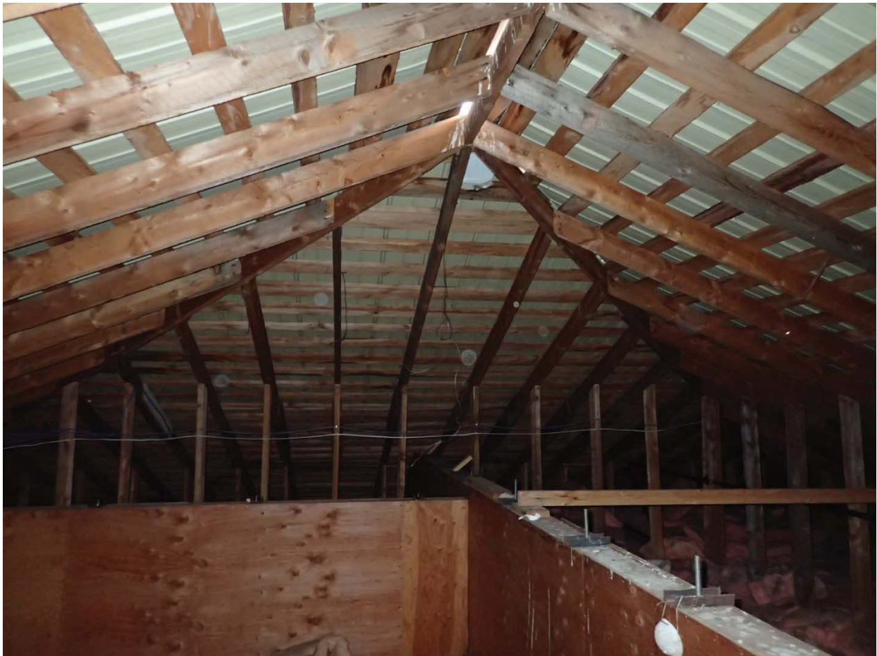
Photo 2: Roof framing viewed from the attic. Note the struts visible in the background.
