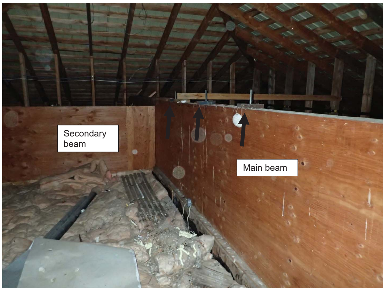
Photo 5: Beams viewed from the attic space. Note the black roofing tar visible on the floor still present on the original school roof area. Some rod locations have been indicated with arrows.
