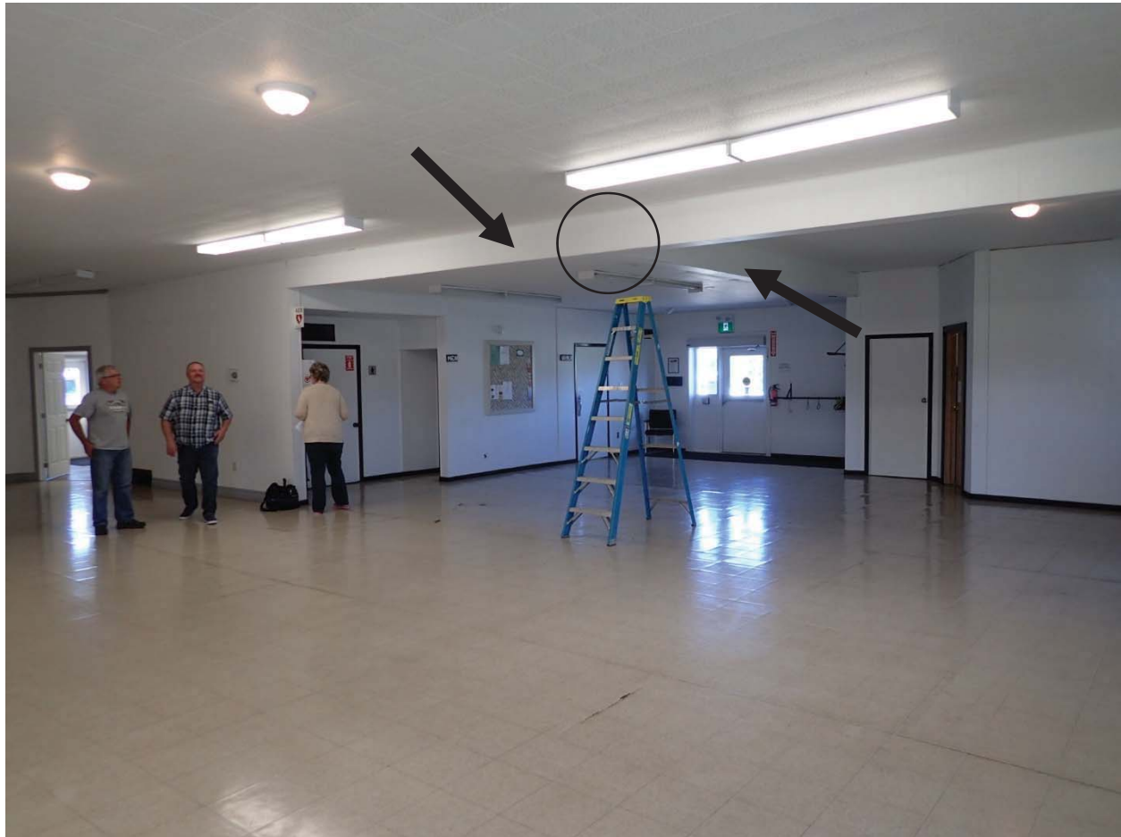
Photo 4: The main hall area. The two bulkheads are denoted by arrows; the area where finishes were removed is denoted by the circle.
